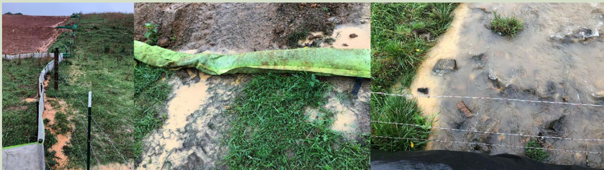
From left to right: Failed erosion and sediment control along the MVP route in Giles County, Va., during MVP construction in October 2018. Sediment escapes the construction site through failed sediment control measures. A stream is impacted by sediment deposition and increased streambank erosion. Photos courtesy of Mountain Valley Watch
